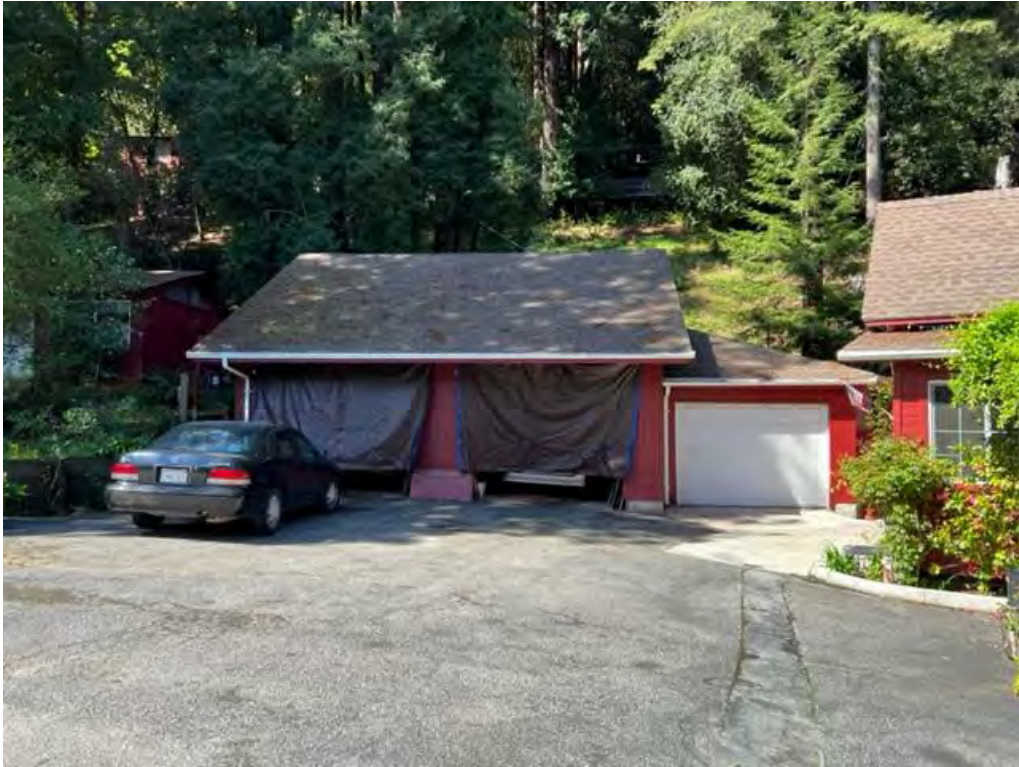
Photograph 5: View looking at the three-car contemporary garage to the left of the manager's office/residence.
