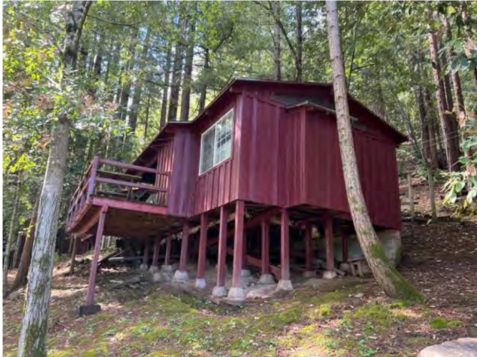
Photograph 17: View of the raised substructure of the upper cabins located on the slope above the lower cabins.
